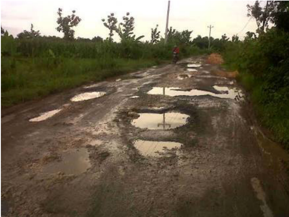
Figure 6. Road conditions damaged in mendenrejo village Kradenan District, Blora Region
