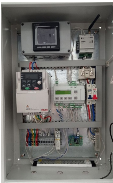
Figure 1. A general view of the control cabinet
