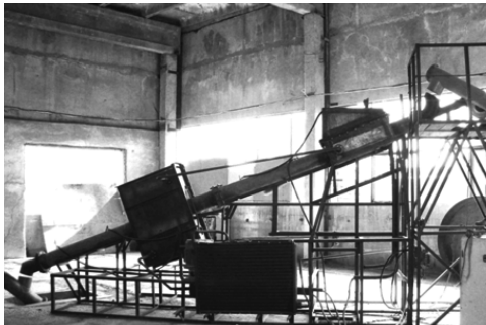
Figure 1. Industrial plant SDSF
