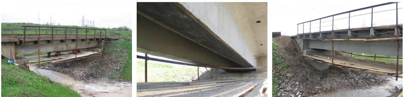
Figure 3. Technology of application of the system of external reinforcement and reinforcement with polymer composite materials
