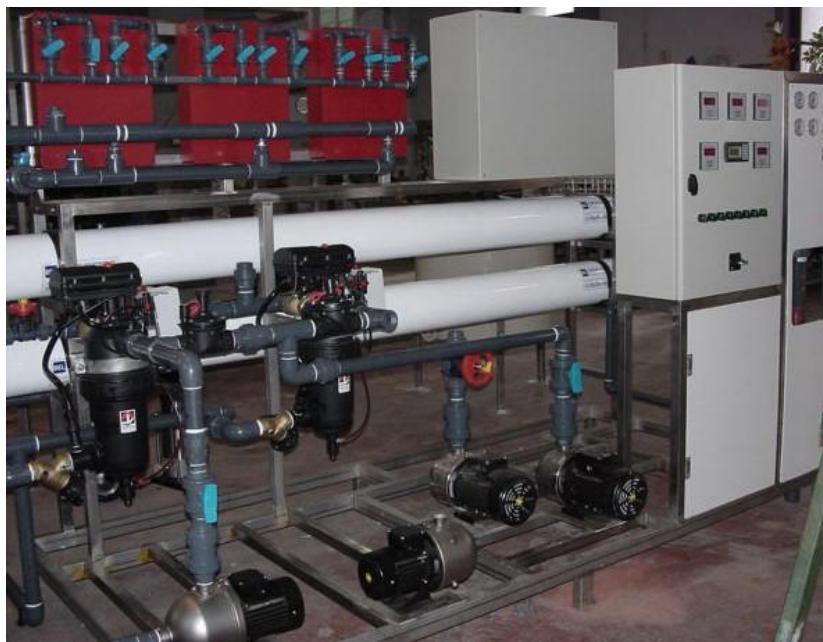
Figure 1. Shows such an innovative installation for treatment, purification, and regeneration of wastewater
