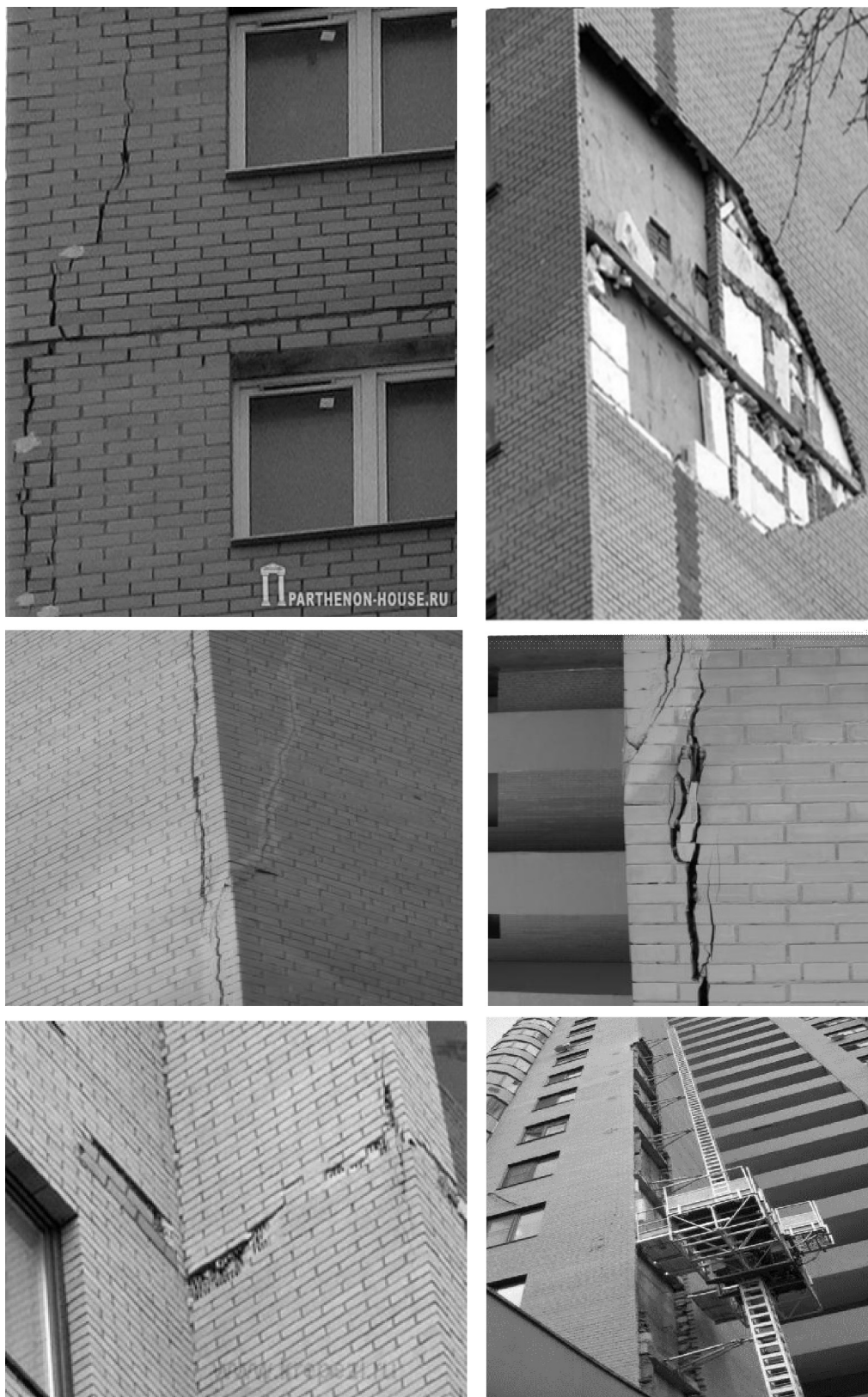
Pic. 1. Demonstration of problems with multi-layer brick facades [6]
