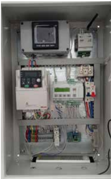
Figure 1. A general view of the control cabinet
