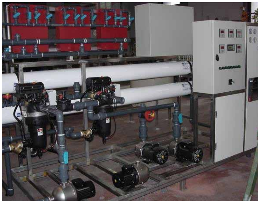
Figure 1. Shows such an innovative installation for treatment, purification, and regeneration of wastewater
