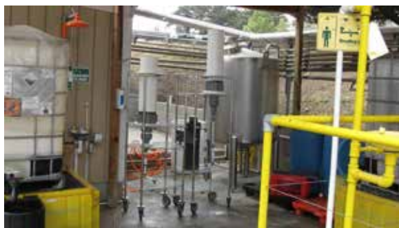
Figure 4. Example of the experimental integration of an innovative system for re-generation of process water without the use of chemical reagents into a typical modern food production facility
